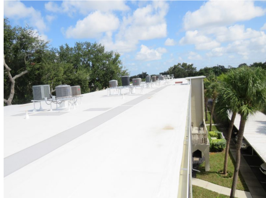
Membrane Roof Covering
